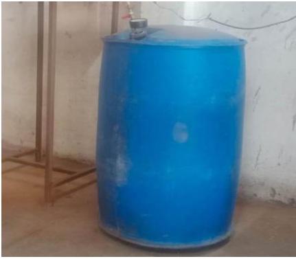
Fig 3 Digester tank during Digestion
